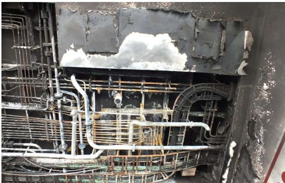
Photograph No. 32. Damaged hydraulic system pipelines
