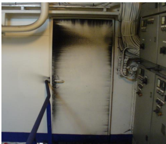
Photograph No. 43. Charred door in the electric equipment room
