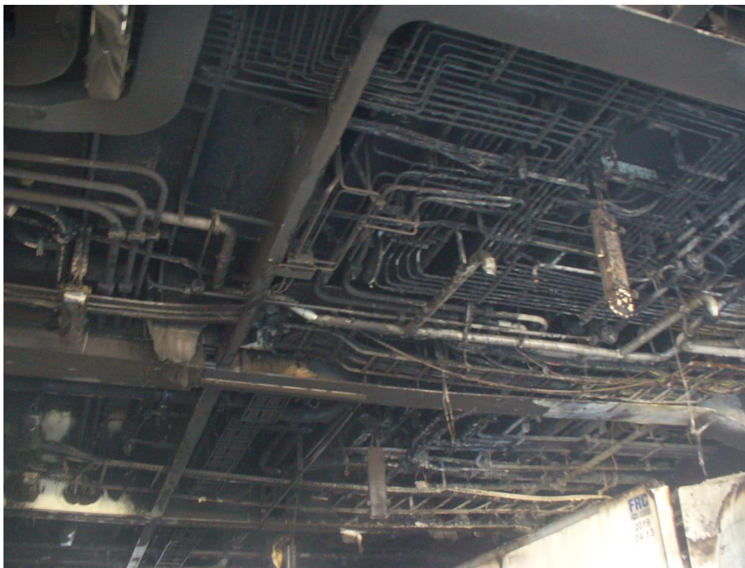
Photograph No. 45. Hydraulic system pipelines routed under the ceiling
