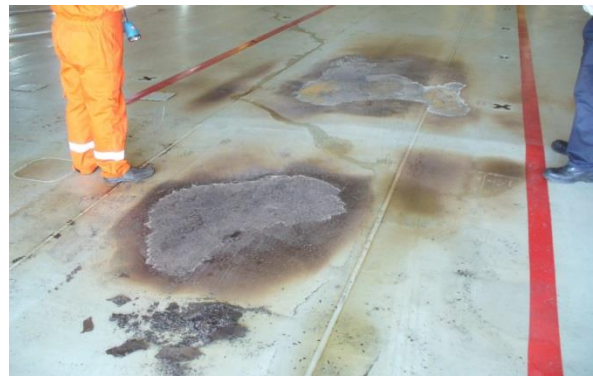
Photograph No. 18. Car deck no. 5; burnt paint spots and deformed deck plate
