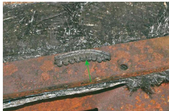
Photograph No. 31. Charred portion of the V-belt
