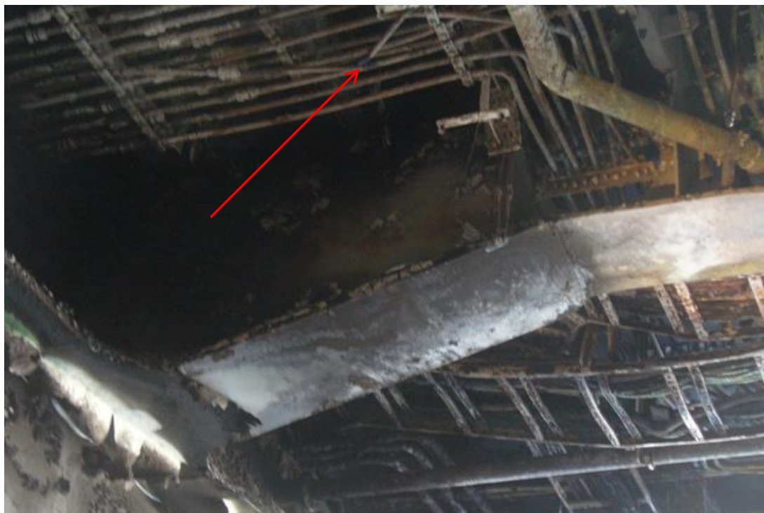
Photograph No. 33. Hydraulic pipeline cracked and deformed as a result of the fire
