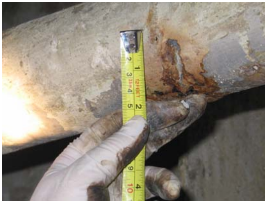
First hole found in pipe leading from Windjammer booster pump going to incinerator room.
