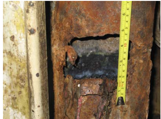
Hole in overboard pulper pipe. Length approximately 3 inches.
