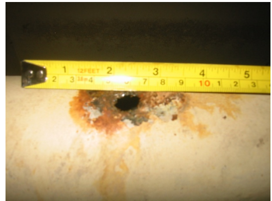
Second hole found in pipe leading from Windjammer booster pump going to incinerator room
