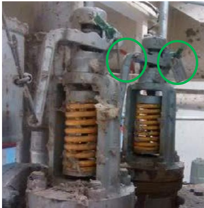
Figure 6: Pressure safety valves – boiler #2, seals ringed in green (source: Brazilian Navy)
