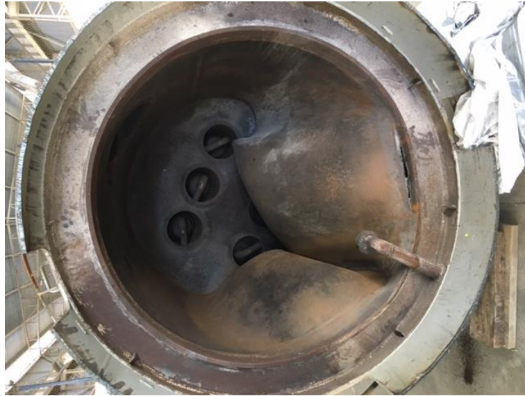
Figure 3: Deformation of internal wall
