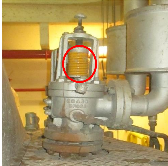
Figure 5: Pressure safety valves – boiler #1 – note compression of spring, ringed in red
