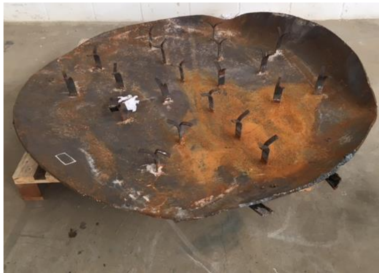
Figure 4: Furnace bottom plate (insulation removed)
