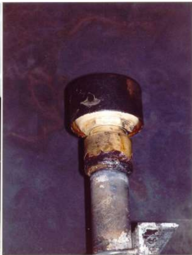
Photos 1 & 2. Deck hydraulic system reservoir tank vent pipe in upper part of engine room
