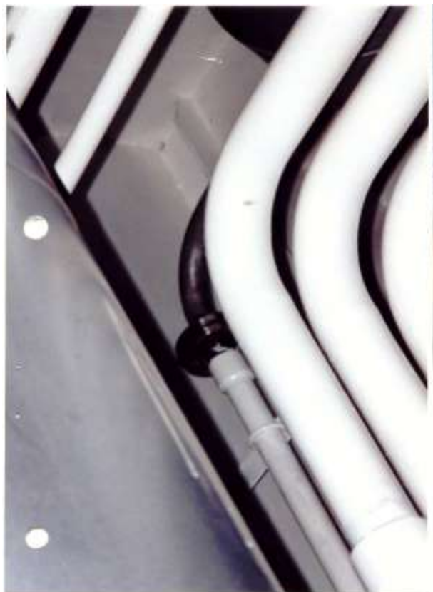
Photo. 4 Deck hydraulic system reservoir tank vent pipe extended up into funnel.
